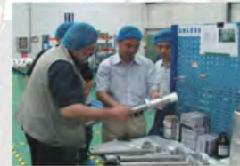
希腊客户参观思源电气SF6断路器装配车间 Customer from Greece had an inspection in Sieyuan
