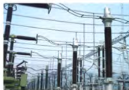
LVB-550 油浸式电流互感器在浙江省电力公司运行 LVB-550 Oil Immersed CT in Zhejiang Province
