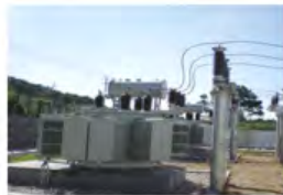
BKS-60000/35 油浸并联在安徽省电力公司运行 BKS-60000/35 Shunt Reactor in Anhui Province
