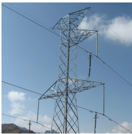
Transmission line arresters
