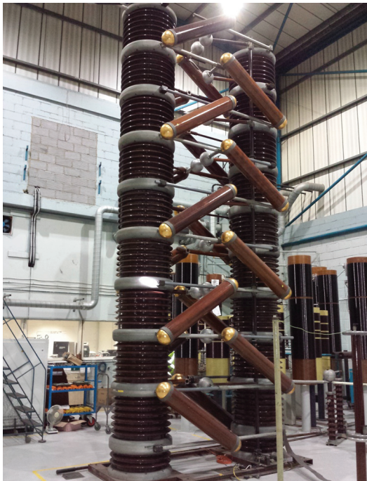
MARX impulse generator 1.65 MV
